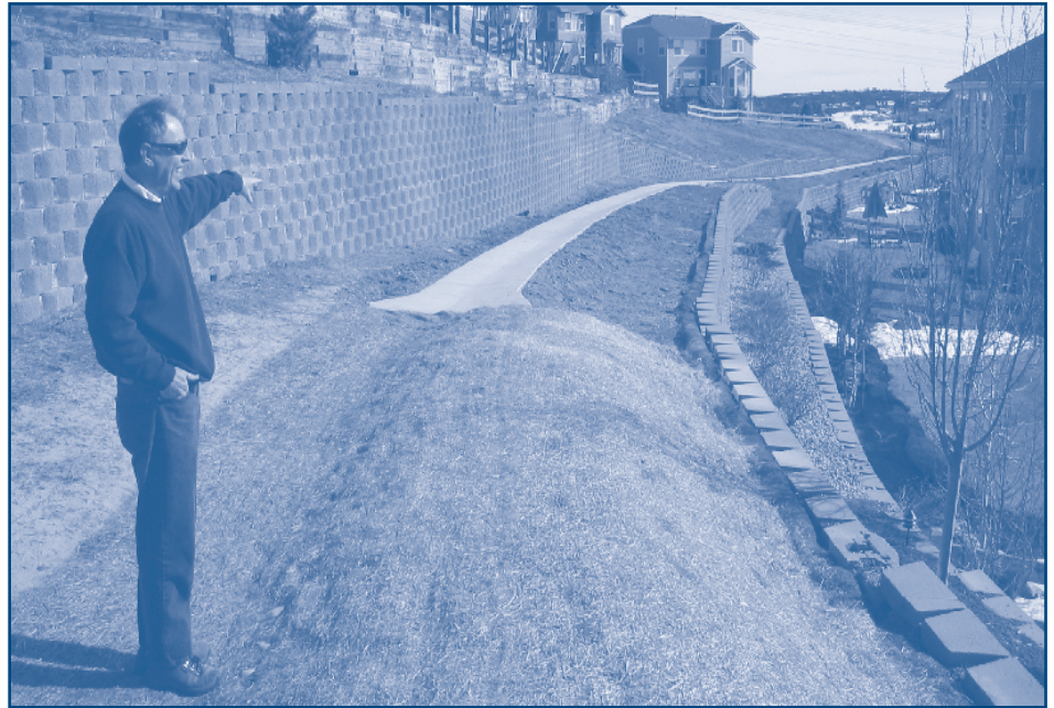
Castle Pines North Metro District Parks and Open Space Manager Charlie Fagan stands on the berm to show how the v-pan diverts runoff behind Arco Iris Lane.
